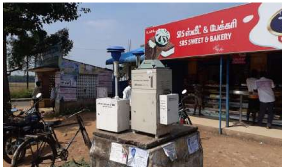
AAQ station at Alinjivakkam (section 2)
