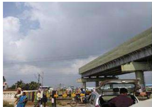
View of an ongoing ROB construction (700m away from the proposed ROB km 55/400)
